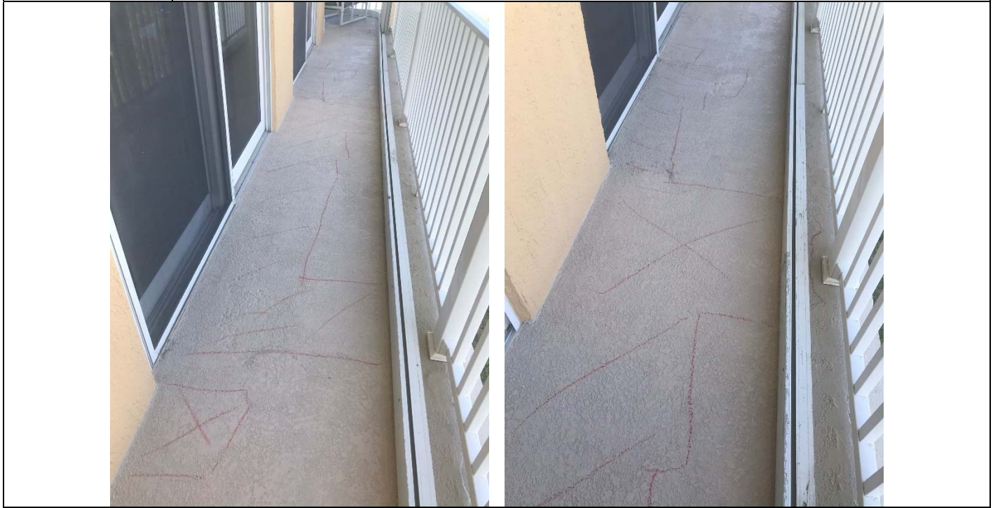
Picture No.: 10,11 DESCRIPTION: Unit 3206: Concrete slab hollow sounding locations.
