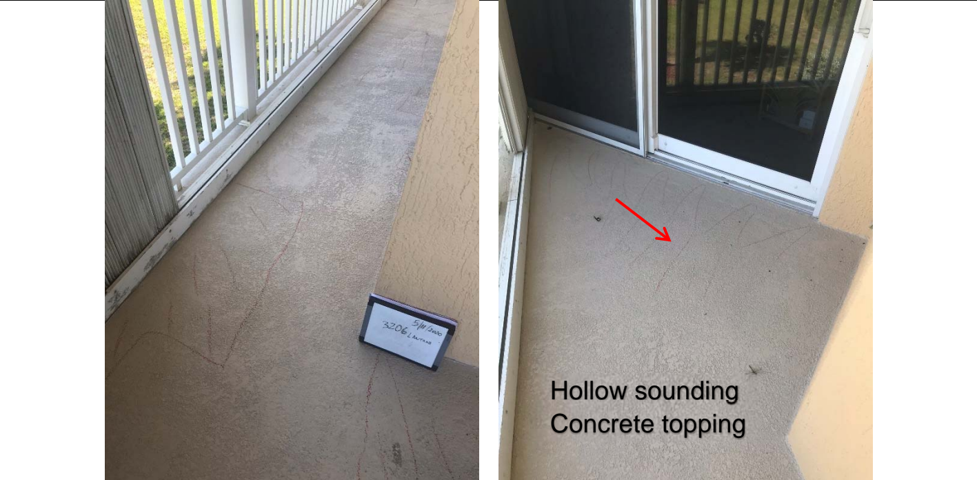
Picture No.: 12,13 DESCRIPTION: Unit 3206: Concrete slab hollow sounding locations.
