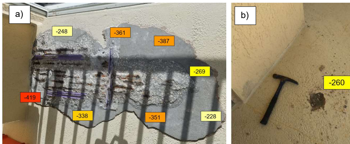
Figure 3: Corrosion Potential Measurements in Unit 3201 Balcony: a) Spall in Front of the Balcony Doors, b) Delamination in Front of the Northeast Column
