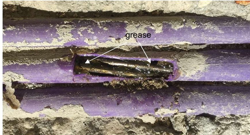
Figure 6: Opening in the Tendon Sheathing
