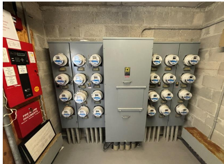
Figure 7: Typical Electrical Panels
