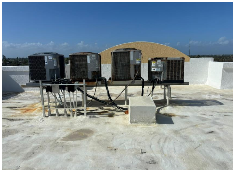
Figure 3: Mechanical Equipment on the Roof
