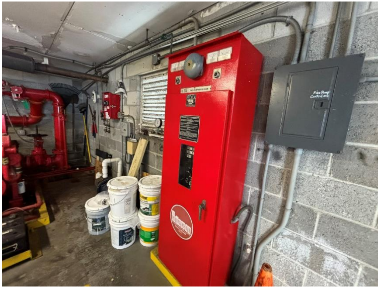
Figure 5: Fire Pump Controller
